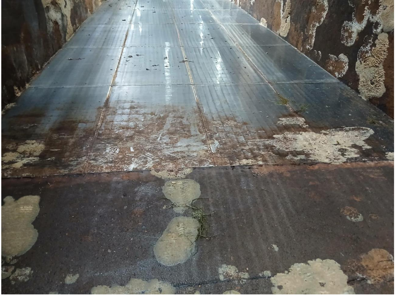
Channel Rectangular Screen along with Walls and Floor
